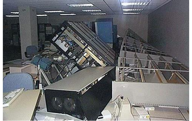
Abb. 2.21.2 &gt; Umgekippte Computerracks
